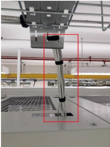
Figure 1.3 Cable dropping to cable inlet
